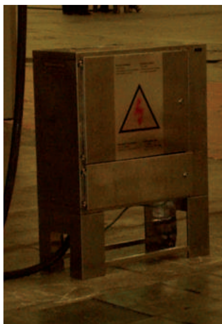
ELECTRICAL BOX (power > 20kW)
