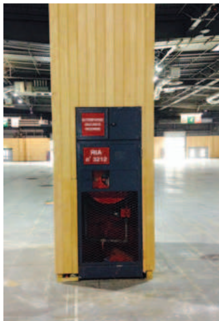
FIRE HOSE CABINETS – RIA (example for pavilion 3)
